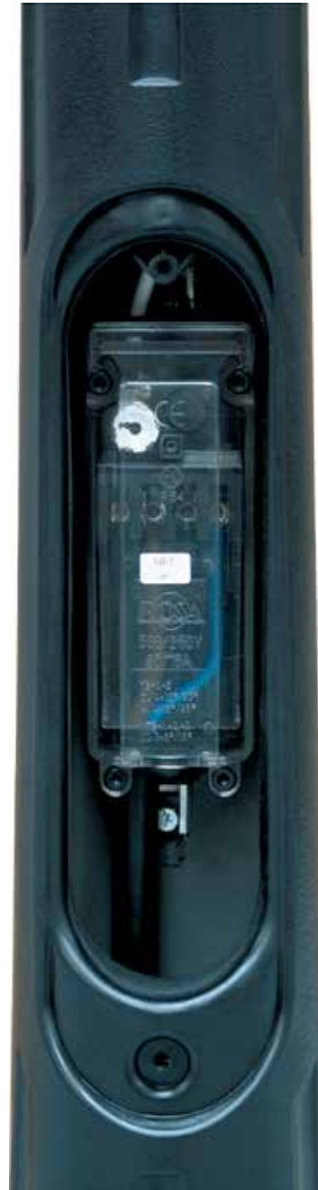
Connection box installed in plastic coated pole
